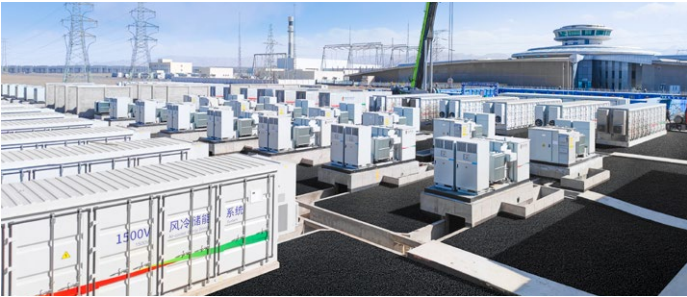
国家电投集团中国电力新源智储青海格尔木共享储能电站项目 100MW/200MWh SPIC China Power XYZ Storage Qinghai Golmud Shared Energy Storage Power Station Project 100MW/200MWh
