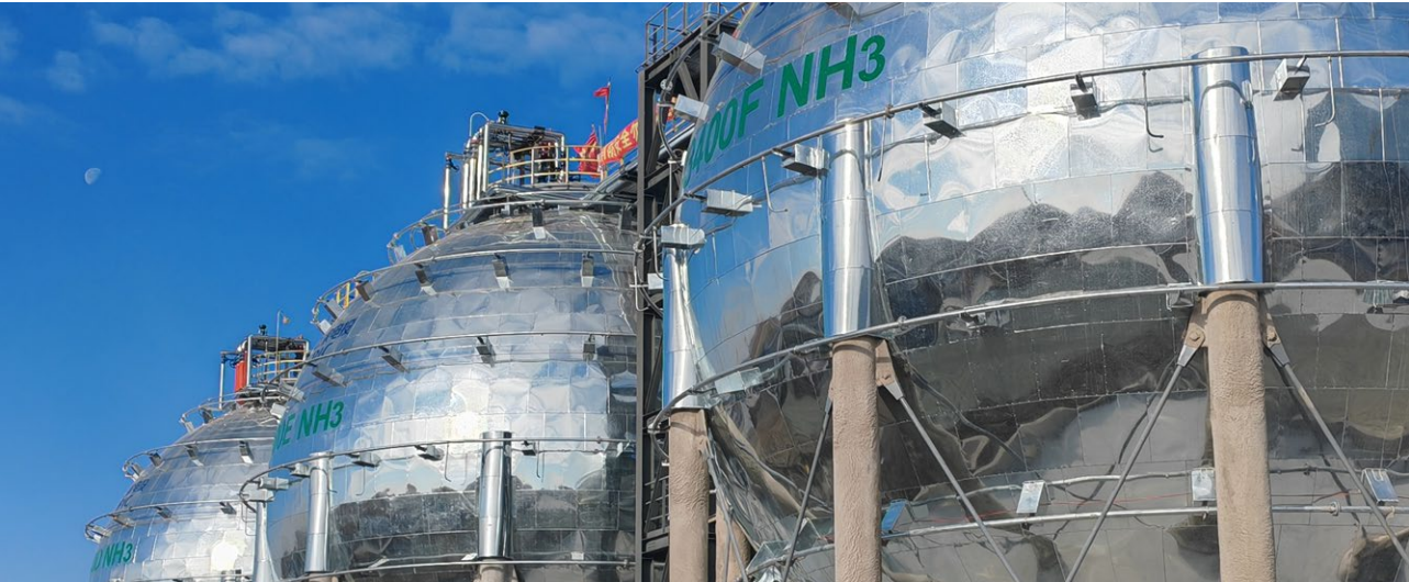
国家电投集团吉电股份大安风光制绿氢合成氨一体化项目液氨球罐 Liquid ammonia spherical tanks at SPIC Da'an Project of Green Hydrogen and Synthetic Ammonia Production with Wind and PV Power
